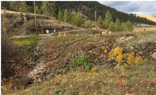
Photo 3: Over-steepened downstream toe to be addressed during the spillway upgrade.
