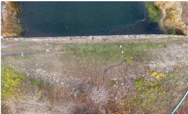
Photo 7: Visible wheel ruts on dam crest.
