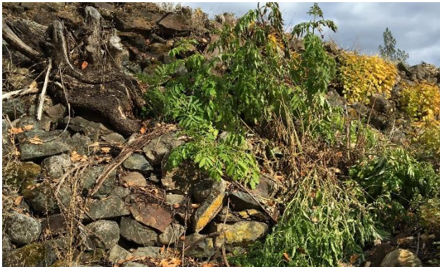
Photo 9: Some vegetation growth noted on downstream east slope which should be cleared.
