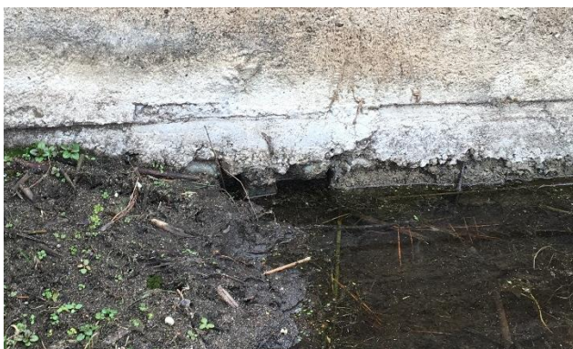
Photo 5: Hole in upstream east side of concrete face of the dam.
