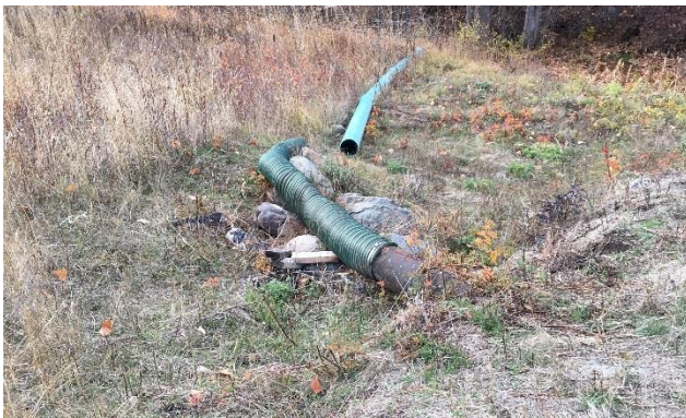
Photo 11: Piping used by the dam operator to diver pipe discharge water from eroding dam. Reconnect piping..
