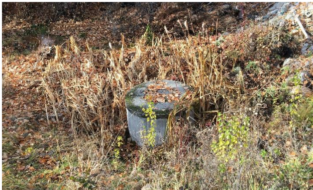
Photo 13: Precast riser structure located downstream of the dam is surrounded by saturated soil.
