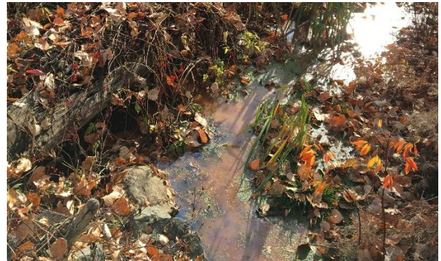
Photo 10: Seepage flow throughout the dam resulting in standing water near toe. Widen the trench width and maintain trench to avoid pooling at downstream toe.
