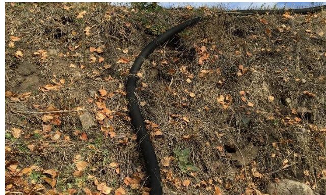
Photo 16: Hose laying across downstream face at approximately the centre of the dam appears to have eroded material off of the downstream face.
