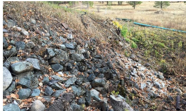
Photo 14: Some raveling of riprap noted on the over-steepened downstream slope.
