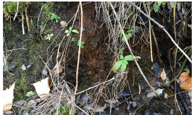
Photo 12: Active seepage noted on downstream east side of dam near precast riser.
