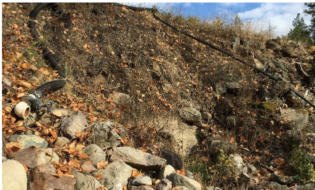
Photo 17: Discharge end of hose (not currently discharging) is located on downstream dam face and should be extended prior to use.
