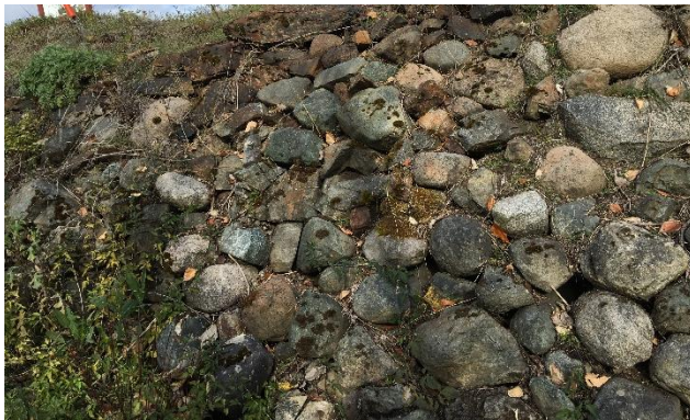
Photo 15: Moss, which noted a previous seepage location on downstream west slope, was dry, likely due to low water level at time of inspection.
